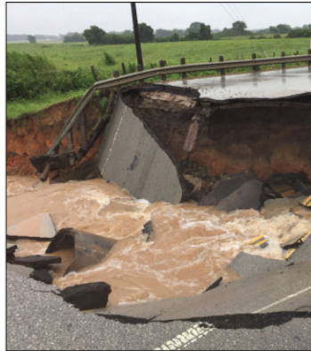
MASSIVE SINKHOLE formed on FM 762 in front of the 24 HR Fitness on Sunday afternoon, making the highway impassable.
