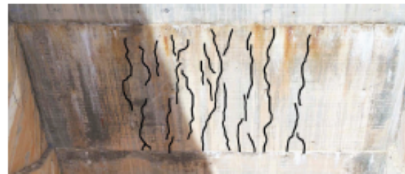
Flexural Cracking Example
