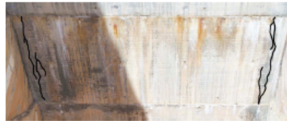
Shear/Tension Cracking Example
