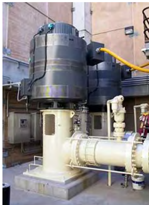
Pictured above: Existing WCRRWL Pumps
