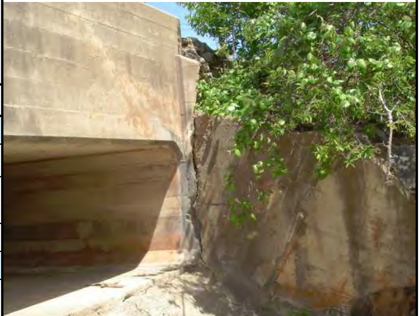
Pictured above: Cracking in the box culvert bridge
