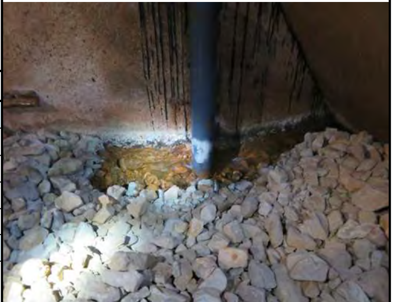
Pictured above: Inside dam within upstream Bay 9 area exposed to leak.
